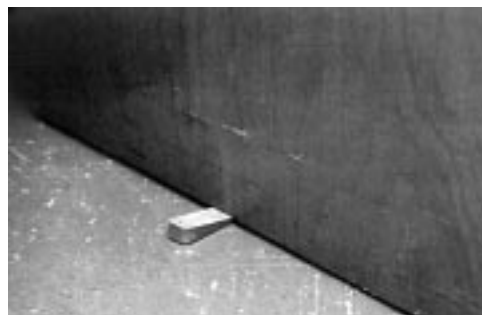
Figure 2 Triangle shaped plastic stopper at bottom of door preventing closure.
